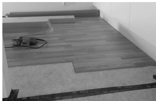
Fig. 1. cTrap installed on the floor with taped seams and edges. New laminate flooring is being installed on top of the cTrap.
